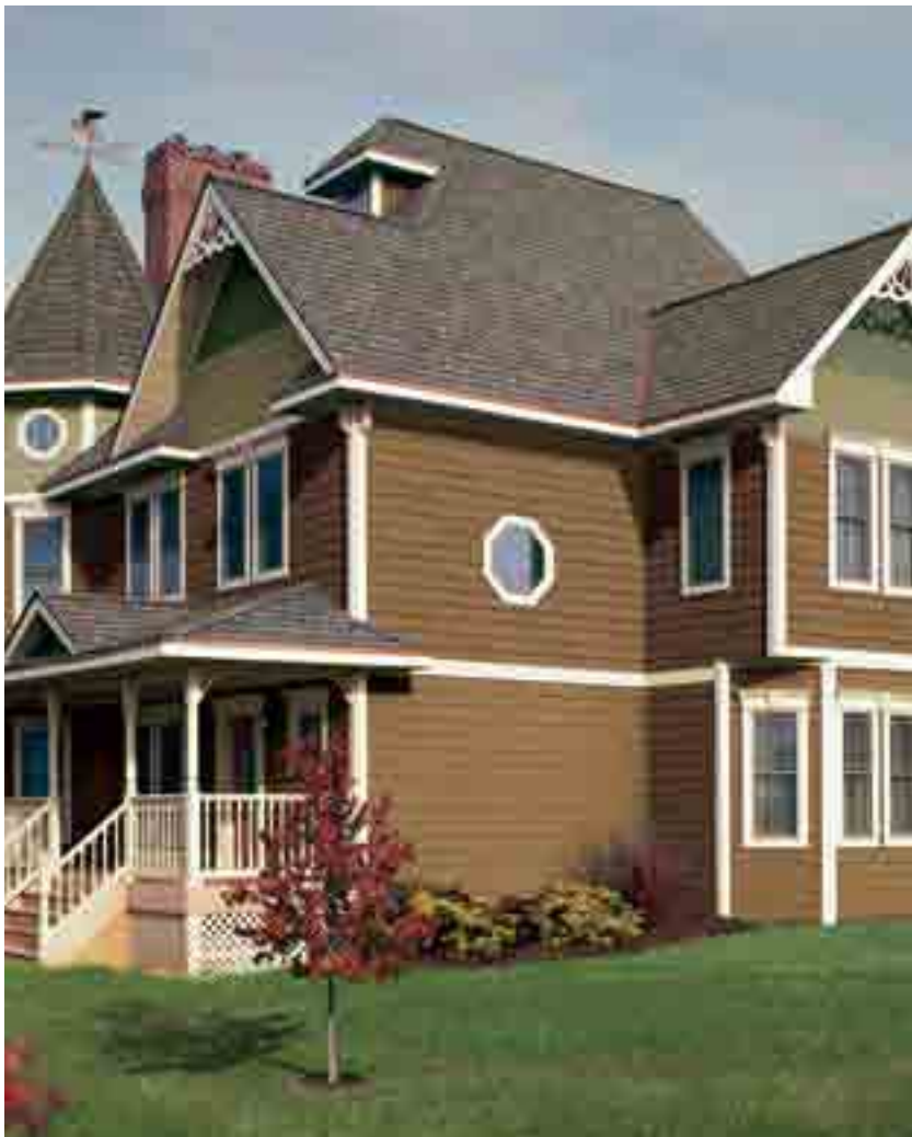
Double 7" Straight Edge Perfection Shingles (1st floor) and Double 7" Staggered Perfection Shingles (2nd floor) in mountain cedar with Half-Round Shingles in spruce and suede.
